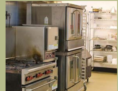
Commercial Grade Kitchen
